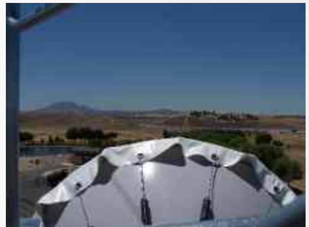
CFIP Full outdoor site
